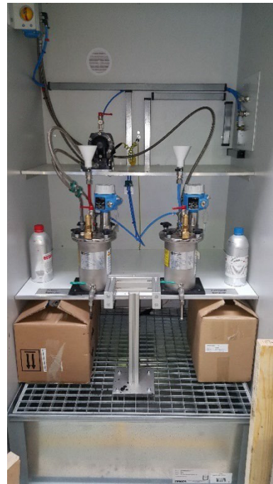
Cabinet for cleaner / primer tank
